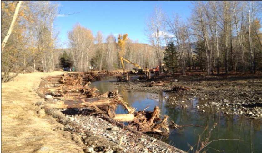
Figure 31. Structures were Added in the Side Channel to Provide Cover from Predators and a Variety of Velocity Conditions for Feeding and Resting.
