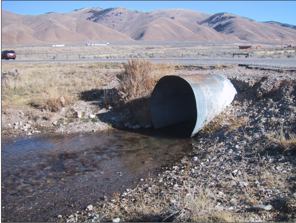
Figure 36. The Canyon Creek Culvert Impeded Adult and Juvenile Passage Before it was Replaced .
