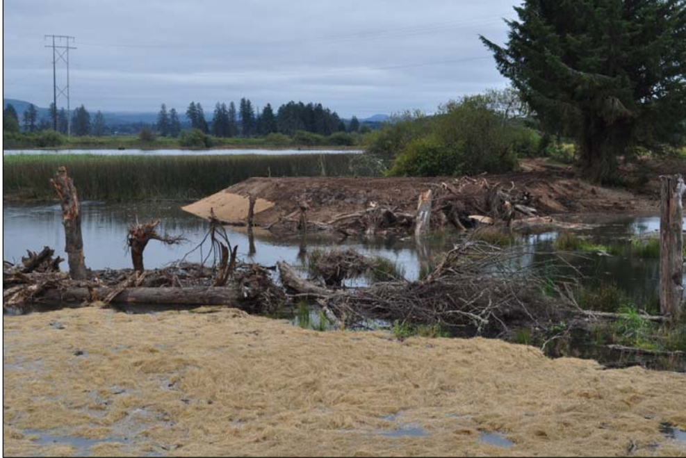
Figure 40. Otter Point as High Tide Inundates the Floodplain Behind the Newly Breached Dike for the First Time in more than 100 years. More than 30 acres were opened for juvenile salmonid use at this project site.
