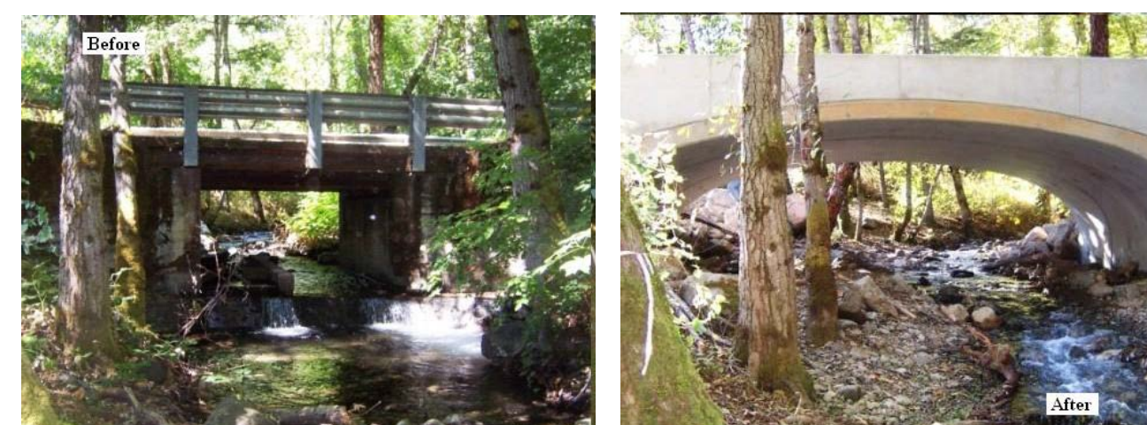
Before and after photos of a 2011 remediated barrier on Conner Creek, tributary to Trinity River, in Trinity County.
